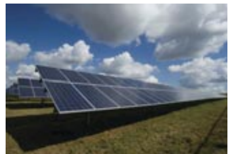
Solar panels line a field in the United States. (Credit: American Public Power Association)
