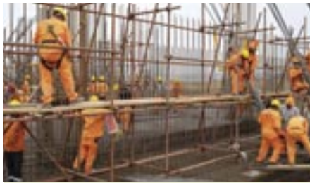
Several hundred workers brought in from China are building the port with Peruvians. Florence Goupil for NBC News
